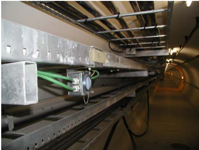
Junction box with signal cabling in ARC
